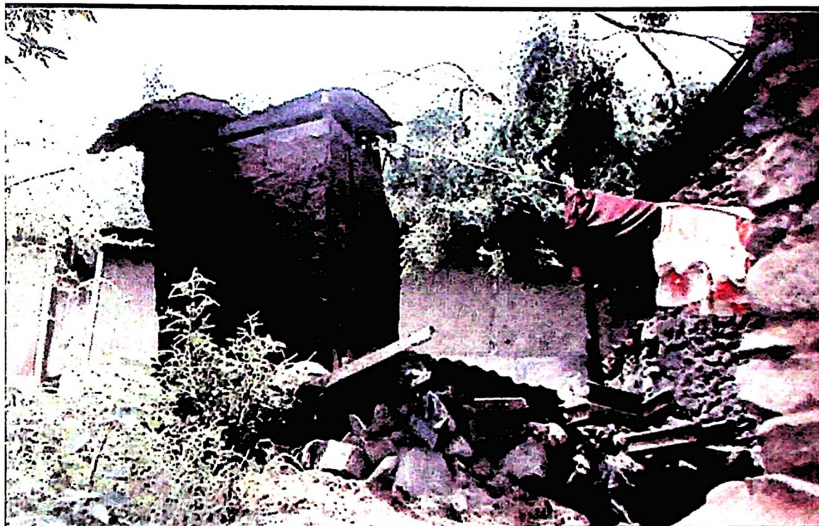
Figure 10: A pour flush pit latrine with a collapsed side pit at Isamilo squatter settlement in Mwanza City
