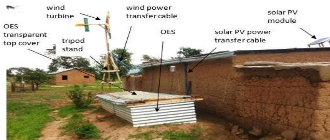
Plate 4.1: The installed i-SWEAD system at the study site (Photo of 11/01/2018)
