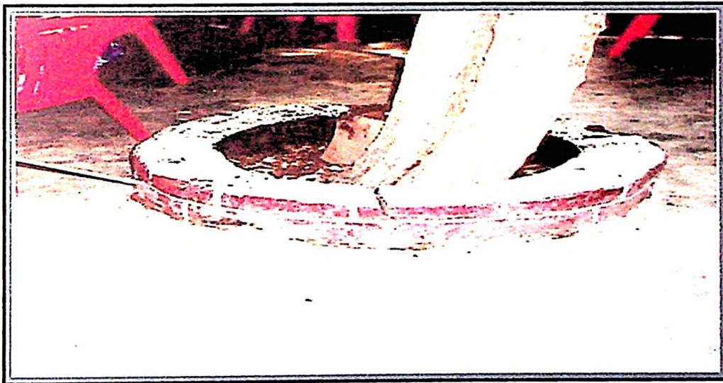
Figure 4: Cracked house floor due to growing Azadirachta indica (Neem) in Kinondoni municipality.
