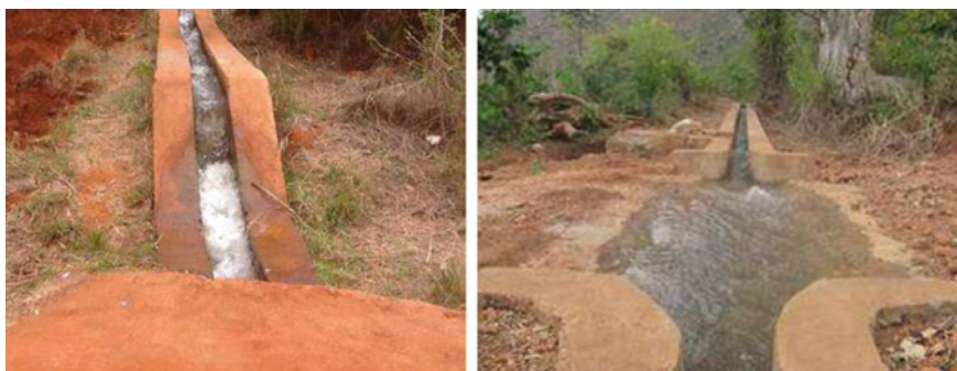
Fig. 5 Improved, lined irrigation canals to transfer water with minimum conveyance losses and shorter time from dam reservoir to field, Bangala, Tanzania. Photographs Sokoine University of Agriculture, Tanzania
