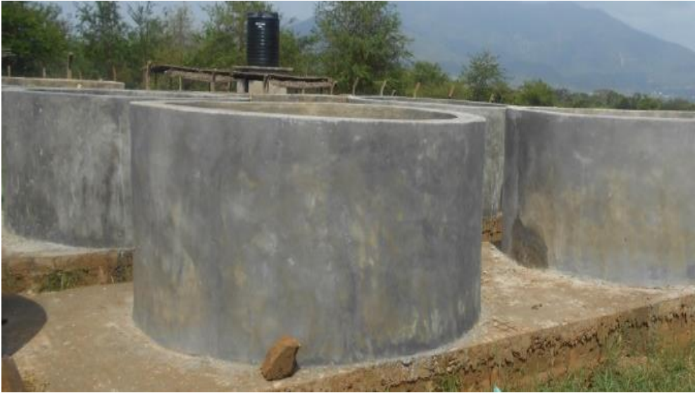
Plate 2: Round concrete tank at Magadu fish farming. Source: Beata (2016).
