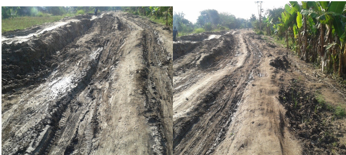
Plate 2: Part of main road that connects study villages (Miwangani, Mpofu and Njage), Ifakara Town, and other nearby villages which was affected by floods in 2014.
